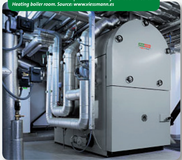
Imagen 1. Detalle de sala de calderas del Distric Heating de Tudela. Fuente: www.viessmann.es | Photo 1. Detail of the Tudela District Heating boiler room. Source: www.viessmann.es
